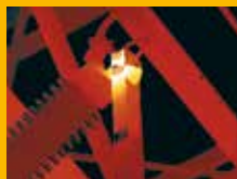
Incorrectly secured connection
