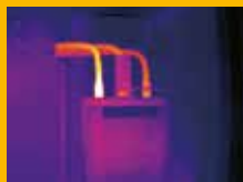
Poor connection and internal damage
