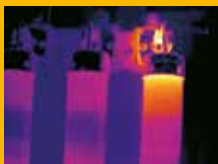
Internal fuse damage
